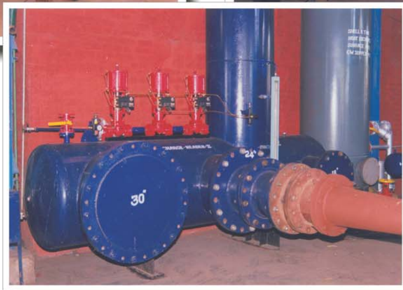
Three numbers of split range control valves installed for very accurate control of discharge pressure of ejectors and thermocompressor under test Break-up, Pick-up pressures are very accurately measured.
