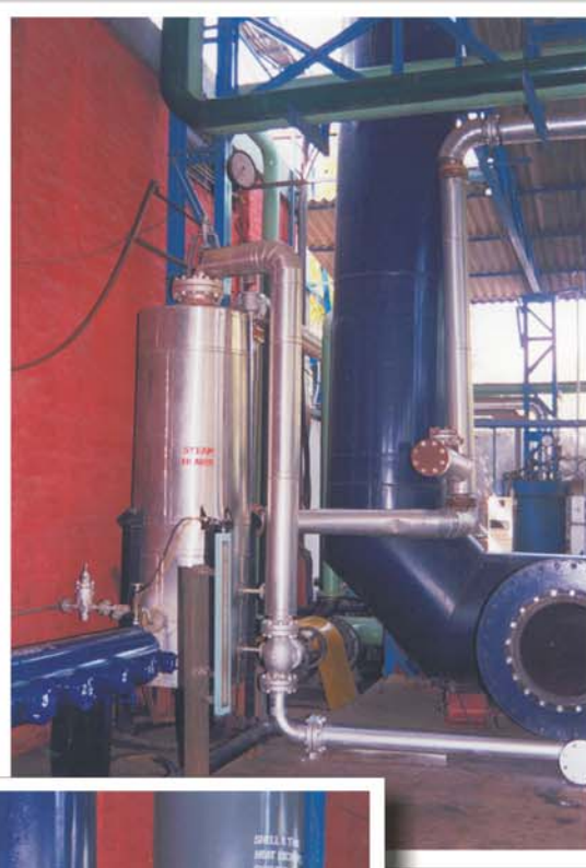
High pressure accumulator to provide additional steam at 17.5 Kg/cm 2 (G) and also at 40 Kg/cm 2 (G).
