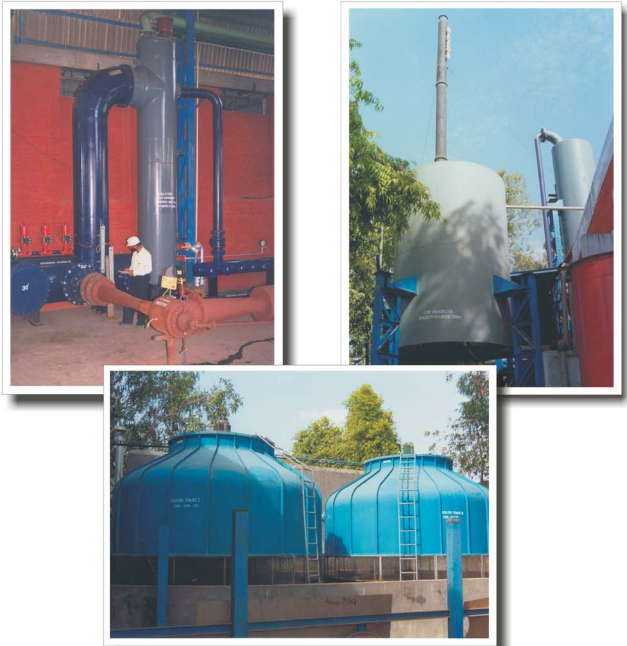
Two numbers of cooling towers having a total capacity of 1200 TR.
