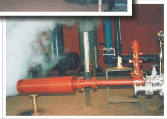
Silencer under test for a start-up ejector to ensure operation at minimum noise level in accordance with OSHA mandated noise exposure limits.
